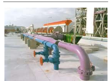
Example of separate piping systems for potable (blue) and reclaimed non-potable (purple) water. Image courtesy of the Water Environment Federation.
